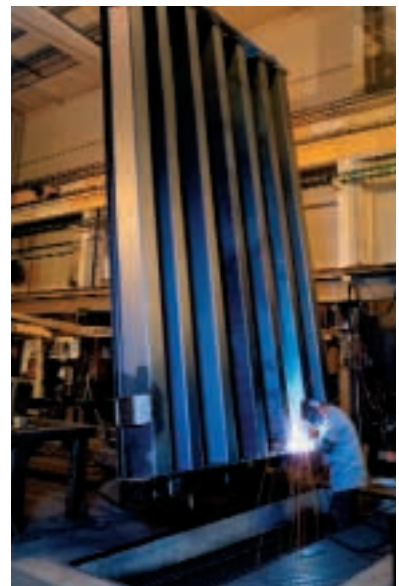
Module positioner allows all welds to be placed in the flat position.
